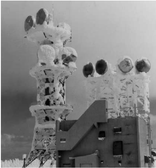
Fig. 5 Snow-stuck microwave antennas on the telephone tower.
