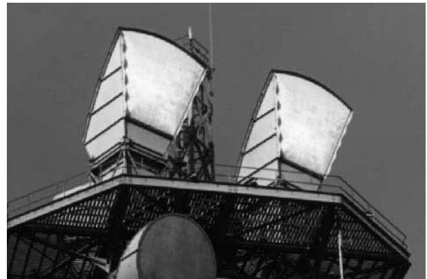
Fig. 6 Horn reflector antennas on the tower.
