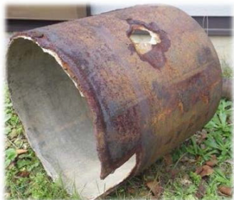
Fig. 3 Water pipe over 40 years old.
